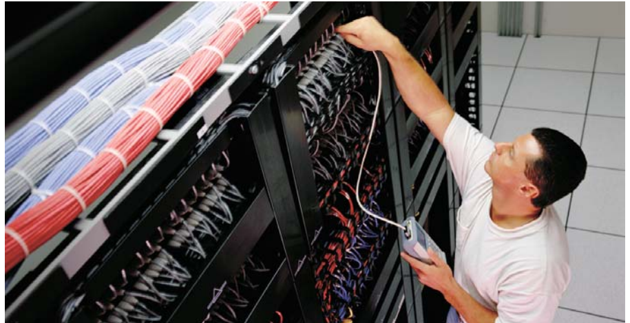
Belden cabling technologies ensure 10 Gigabit performance.
